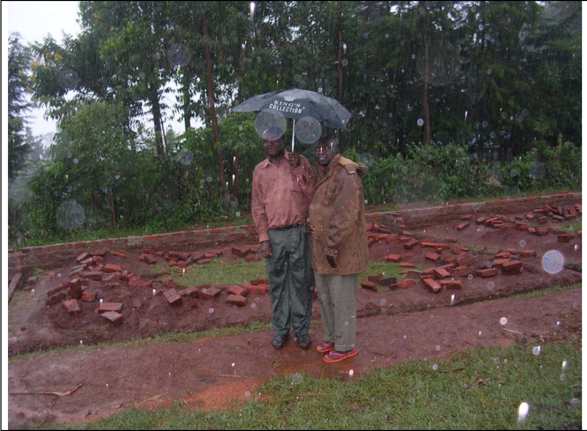
Deputy head teacher braves rain to show Aggrey the site for the new secondary wing
